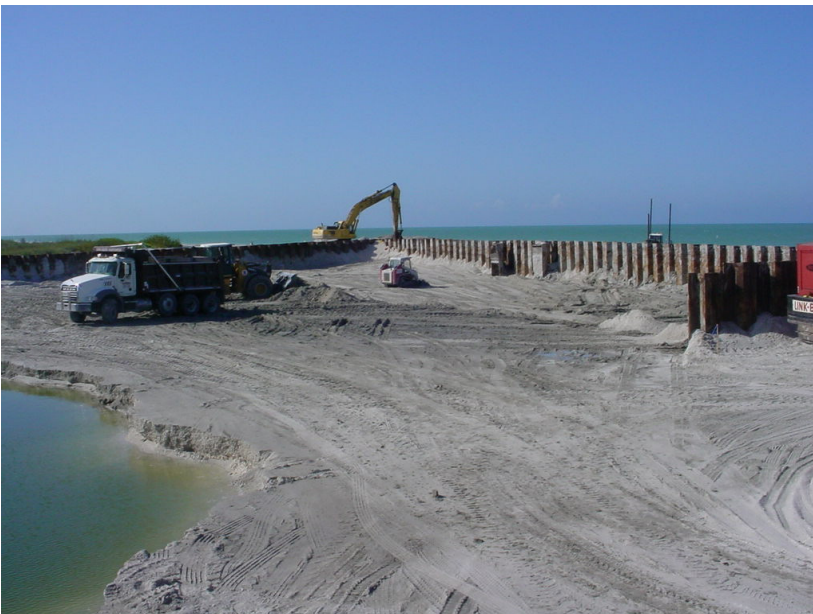
Monday, May 04, 2009 Truck Loading Operations for the Clayey Material at Blind Pass.
